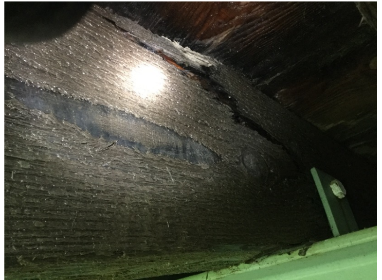
2 cracked ties just outside downstream girder
